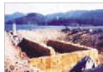
▲ Innovative filtering system to protect water
